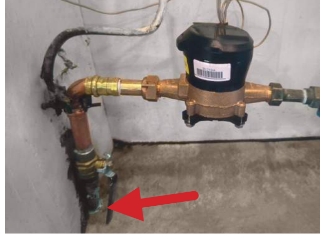
Water service line penetrating the floor
