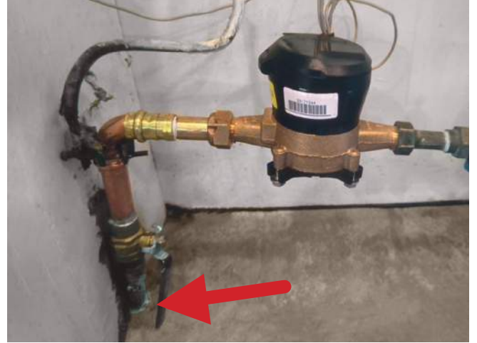
Water service line penetrating the floor
