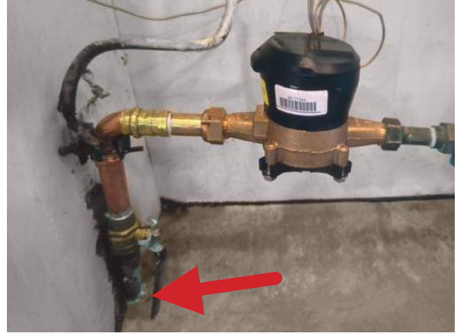
Water service line penetrating the floor
