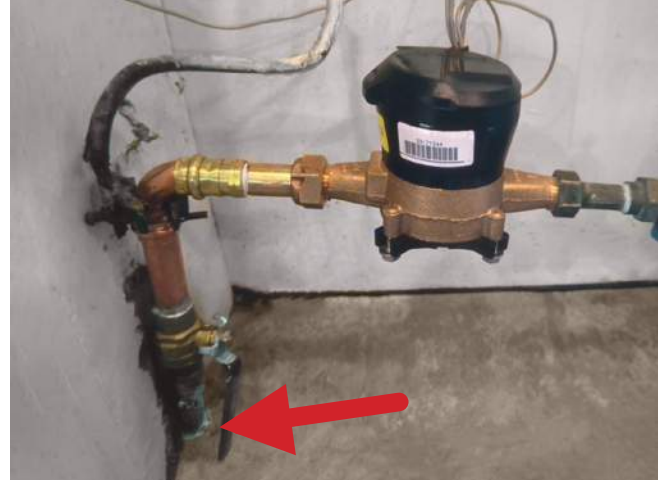
Water service line penetrating the floor
