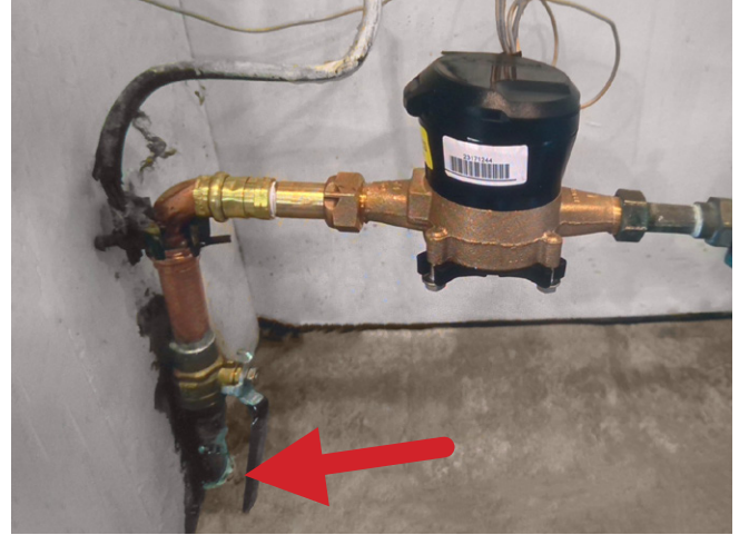
Water service line penetrating the floor
